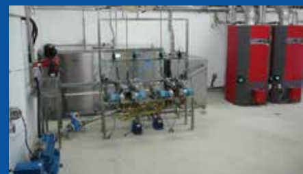
Equipment room solution
